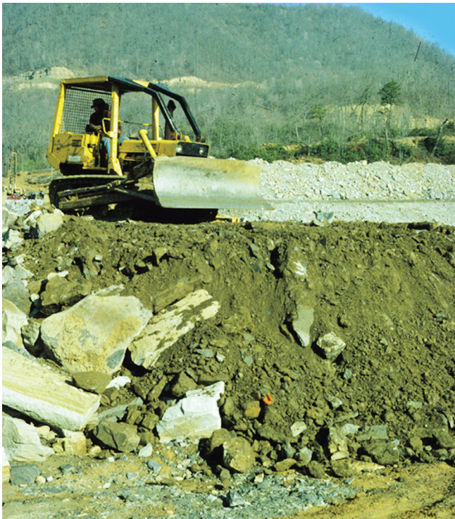
Figure 6. Final reclamation grading of a topsoil substitute. The designated material has been end-dumped in closely spaced piles and is being graded with a small bulldozer. By following the set of practices outlined in this chapter and excluding traffic after final grading, 3 to 4 feet of loose, uncompacted minesoil material can be created in most surface mining environments.
