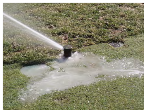
Figure 8. Leaky o-ring identified during routine inspection.
