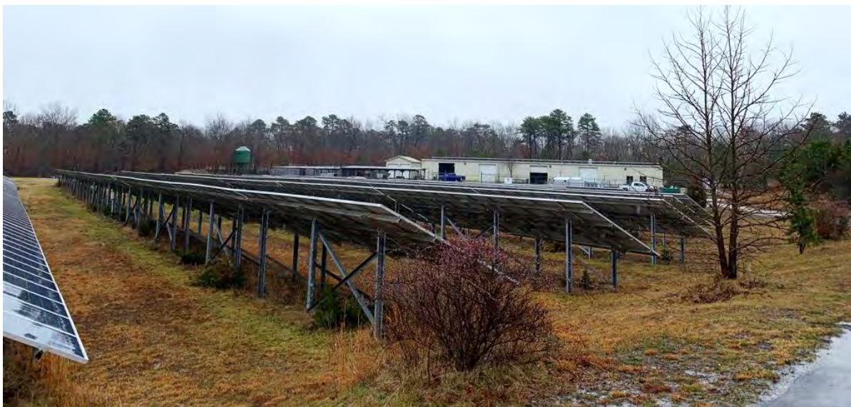
Figure 32. Solar panels installed at a golf course facility can be a renewable energy source.
