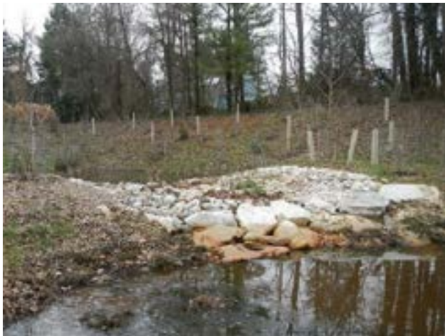
Figure 3. Step Pool Stormwater Conveyance weirs have a cobble apron on the upstream side, reinforced with boulders.
