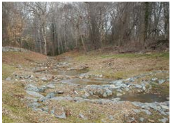
Figure 2. A Step Pool Stormwater Conveyance directs runoff from parking lots to Broad Creek in Annapolis, Maryland.
